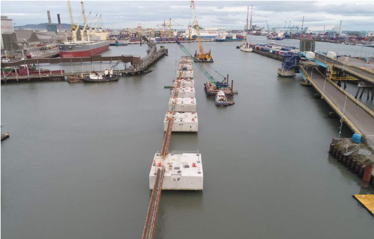
Figure 85. Dublin Port ABR, New RoRo Jetty. Photo courtesy of the Department of Transport, Tourism and Sport
