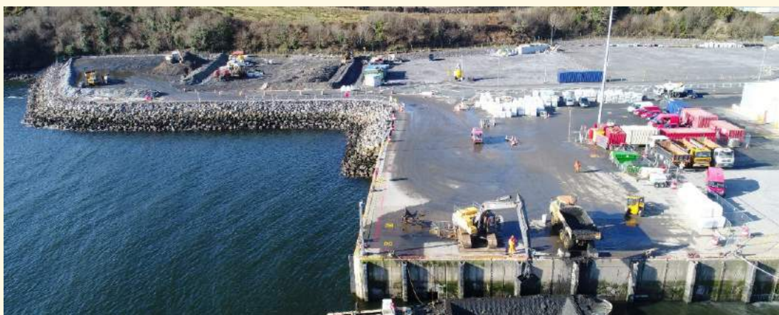
Figure 79. Smooth Point Pier Extension Phase 1 Dredging, Killybegs FHC. Photo courtesy of Department of Agriculture, Food and the Marine (DAFM)
